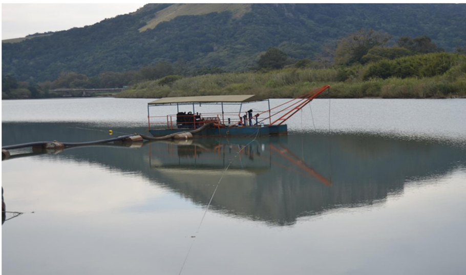
Image 2.5: Example of a small dredge with a floating polyprop pipeline that pumps to a discharge pad
