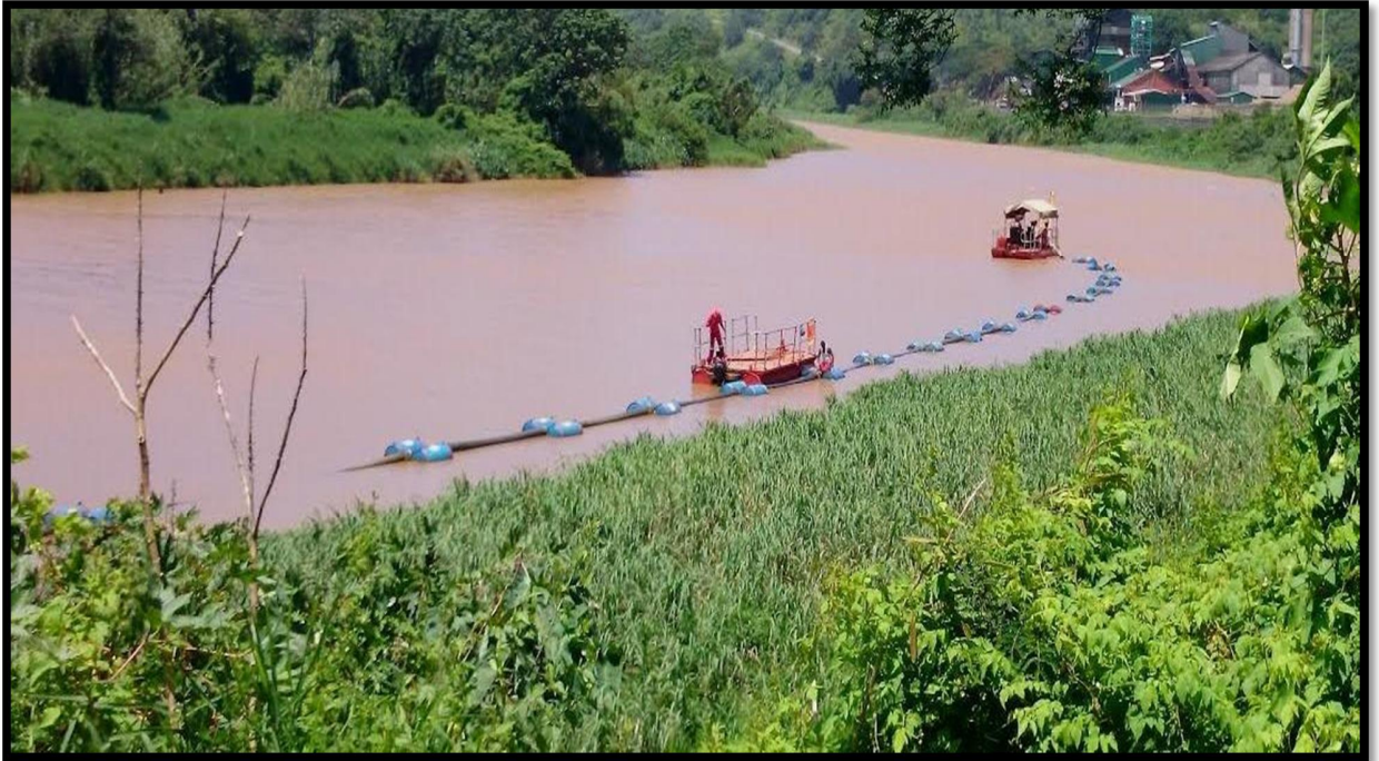
Image 2.2: Example of Floating Barge, Pump and Pipe System
